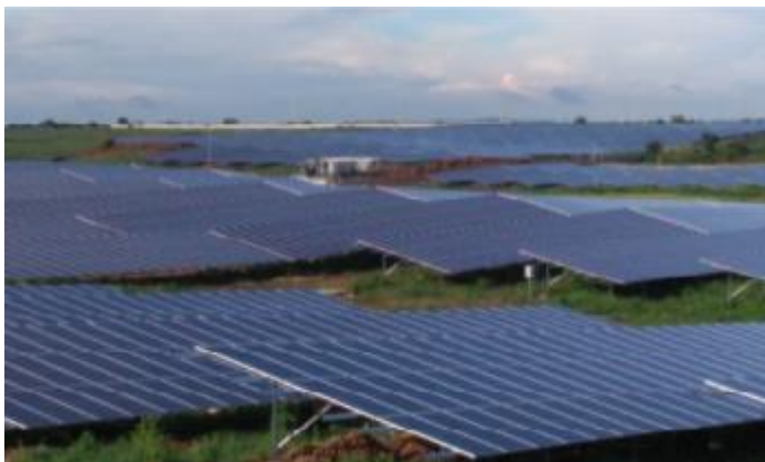
Offsite ground mounted solar plant
